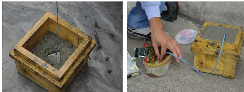
Fig. 13. Preparations to measure early age concrete temperature and humidity using a SHT21S sensor inside a mortar shell.
