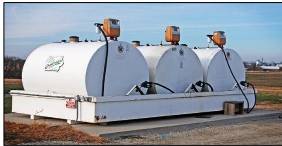
Figure 37 - Fuel tank equipped with a Dike [74].
