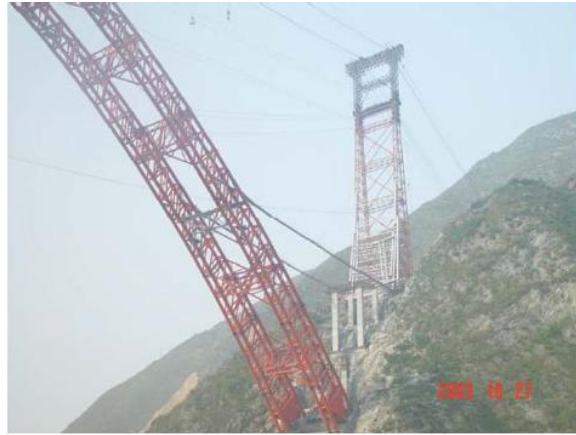
Figure 2.6 Erection procedure by cantilever method in Wushan Yangtze River Bridge (adapted from [1])
