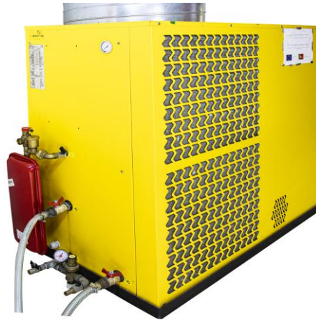
Figure 31 – Picture of the MTA TAE EVO 031 chiller used, with inlet and outlet ports visible on the bottom left corner.
