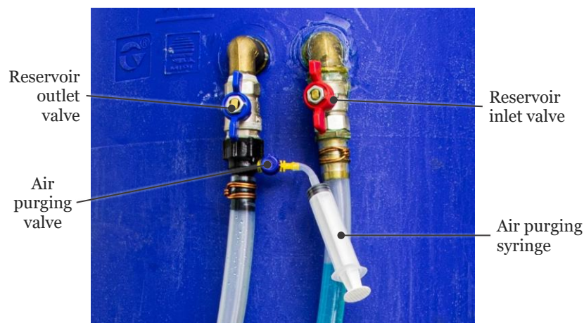
Figure 34 – Picture of valves and air purge system.
