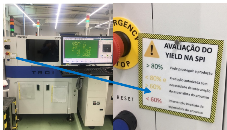
Figura 14 - SPI (Solder Paste Inspection), HFA.
