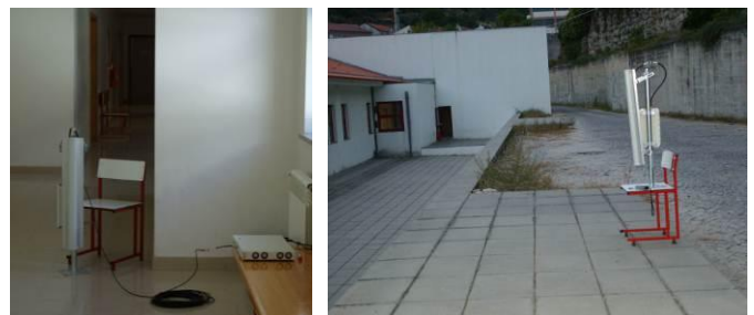
Figure 2. Indoor and outdoor-to-indoor installations with BS sectored antenna
