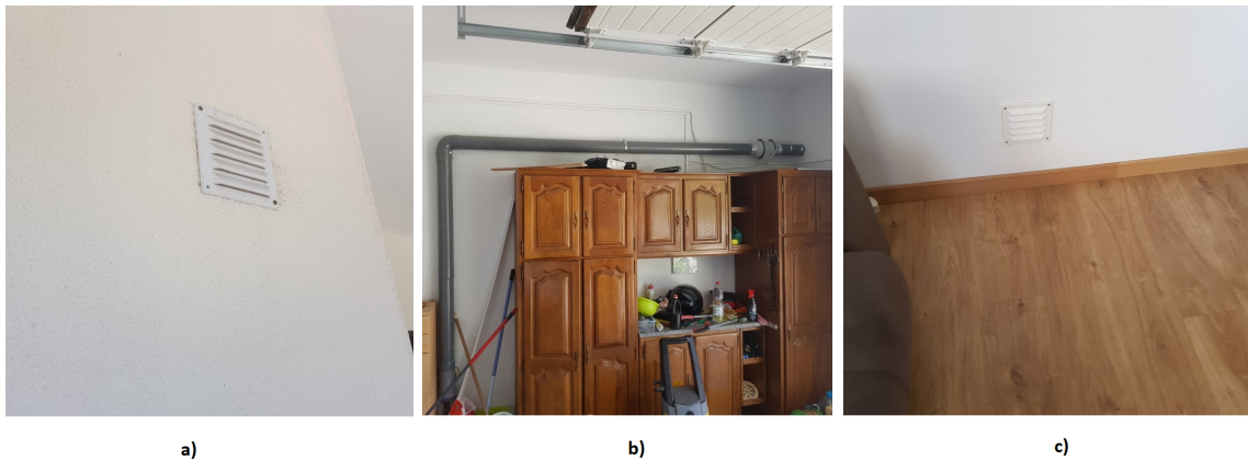
Figure 5.3: Ventilation system installation in the living room- a) outdoor installation b) Installation of tubes and fan c) indoor installation
