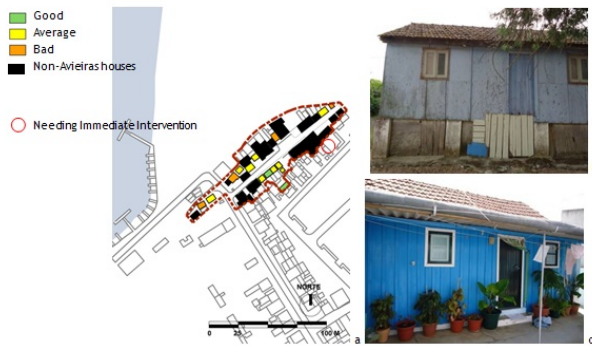
Figure 6: ICT platform application for evaluation of status of wooden stilt-houses conservation, in Escaroupim: a. vernacular stilt-house village of Escaroupim; b. the worst case of status of building conservation (corresponding to the wooden stilt-house no. 1); c. the best case of status of building conservation (the single-story house no. 29a).
