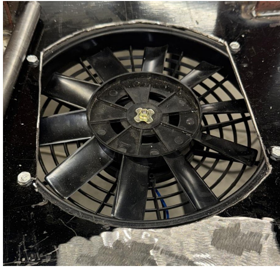
Figure 3.22: Coil and disk cooling fan installed on the ETB table.
