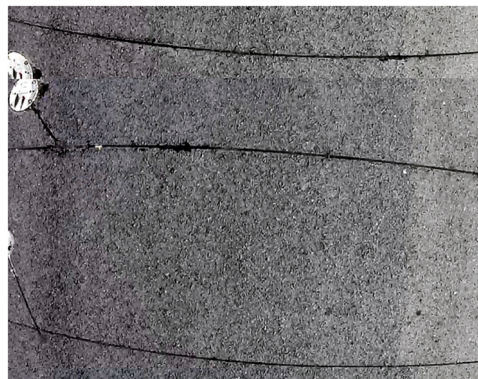
Fig. 5. GIS visualization of part of sample unit 71 with patching and utility cuts distress.
