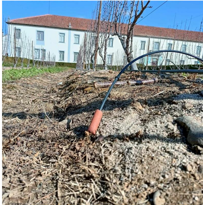
Figure 31. SLECI main line before installation underground, at the moment of the test run
