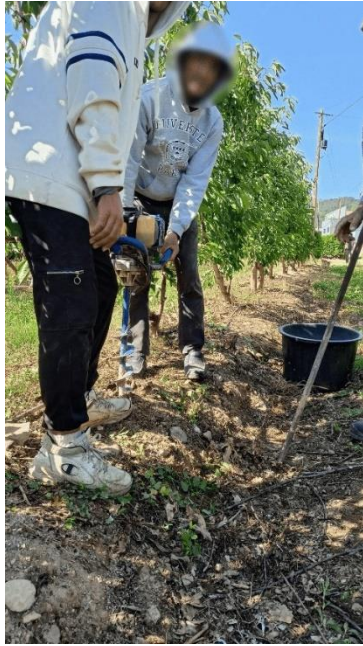
a) Drilling process of the bore hole for the doubling of the SLECI elements
