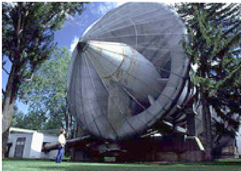
Figura 3.5 - Ventilador do 3mx6m Open-Circuit Propulsion Wind Tunnel. (Fonte: http://www.nrc-cnrc.gc.ca/eng/facilities/iar/propulsion-tunnel/technical.html ).
