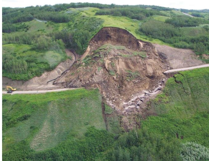
Figure 34. Example of a translational landslide (Bobrowsky & Highland, 2008).
