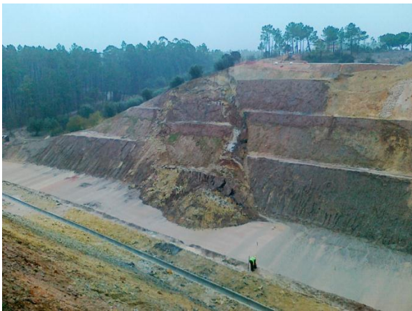
Figure 4. Landslide along Highway IC36, Leiria, Portugal.
