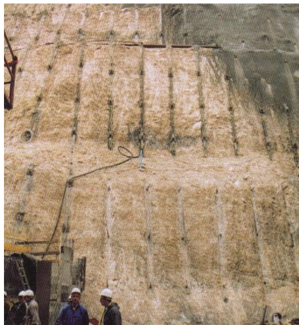
Figure 92. Excavation of a large slope stabilized with tied anchors (Vallejo, Ferrer et al., 2004).
