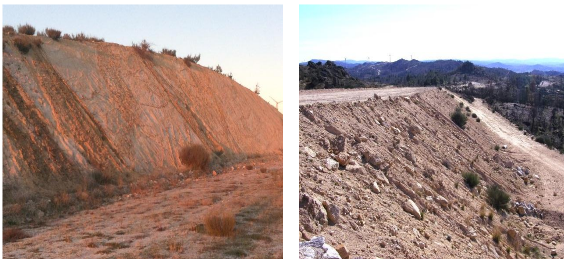
Figure 15. Cutting through granitic residual soils of the Covilhã region and embankment constructed along the same road alignment reusing these materials.
